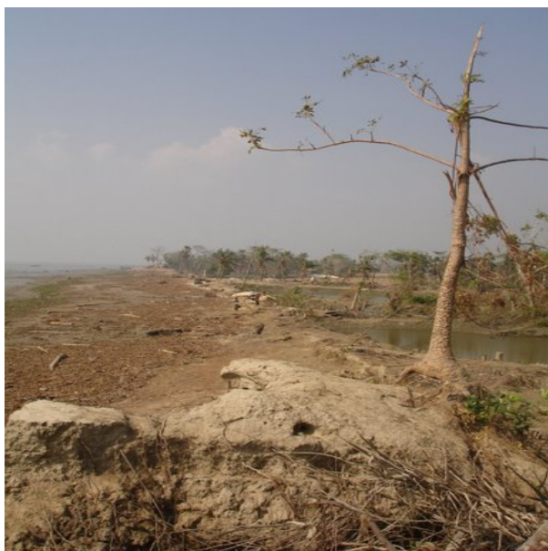
Figure 19: Embankments Washed Away By Sidr's Storm Surge
