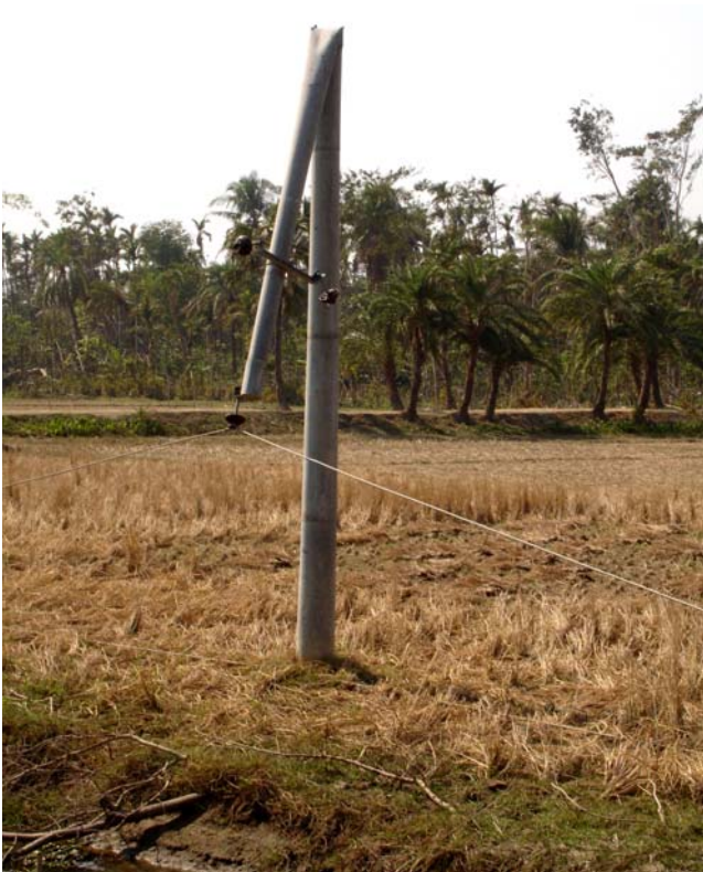
Figure 17: Damaged Power Pole
